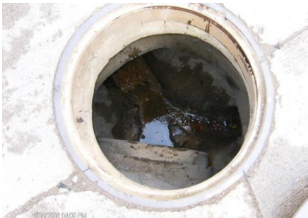
Illegal Sanitary Connection to Storm Sewer System
